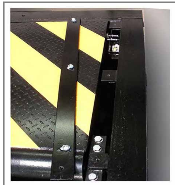
Sideplate removed for access to limit switches.
